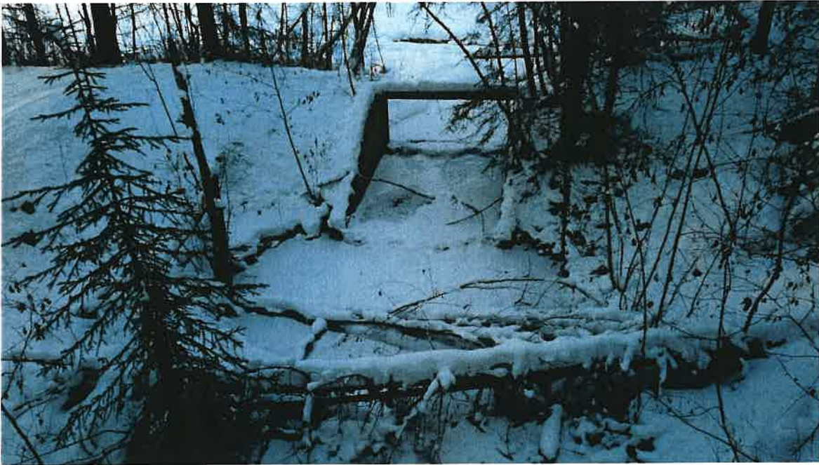
Photo 4 Downstream Side of Concrete Spillway Structure with Woody Debris in Outlet Channel
