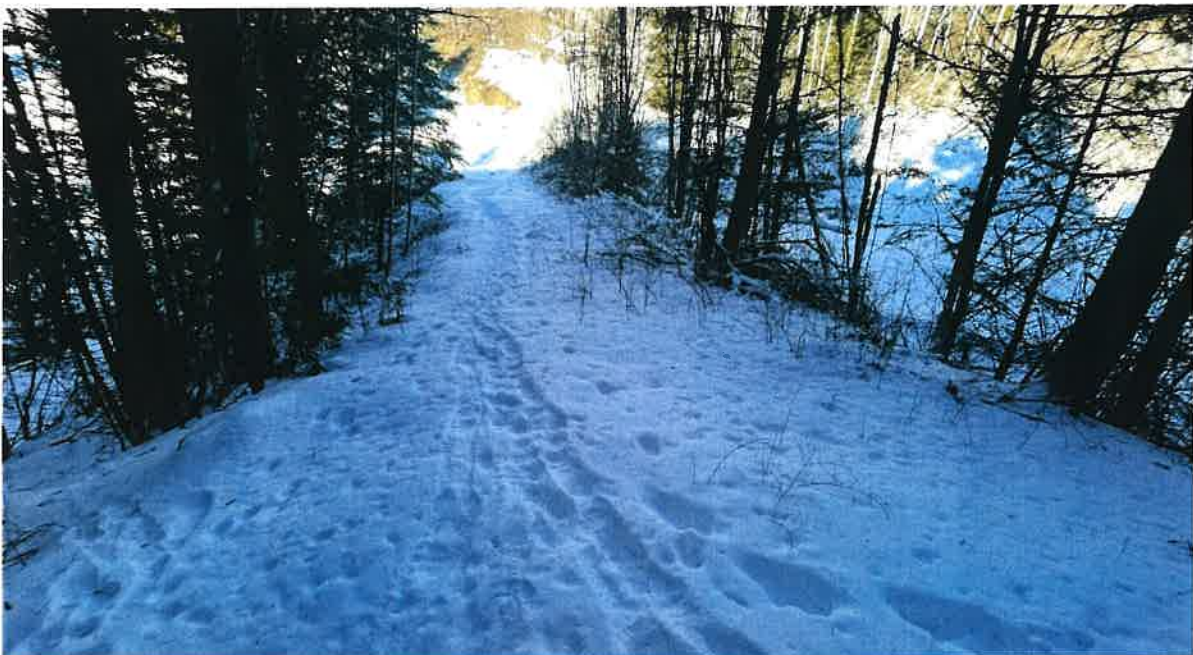
Photo 2 Dam Crest with Trees on Upstream and Downstream Face
